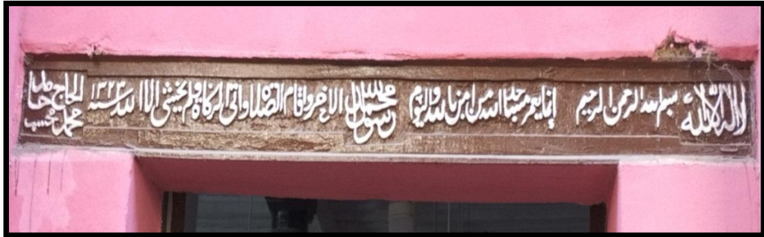
(Pl. 9) The upper wooden lintel of the entrance door on north façade. (Photographed by the author)
